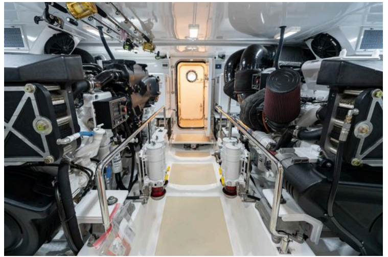
Engine Room Facing Port Aft
