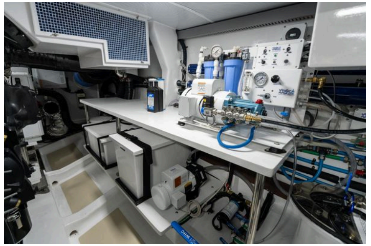
Engine Room Facing Port
