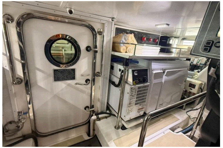
Engine room of 2018 Marlow 53E yacht with equipment and storage shelves.
