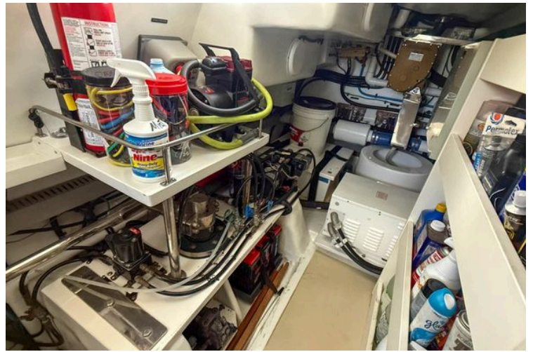
Engine room of a 2018 Marlow 53E yacht, featuring tools and maintenance supplies.
