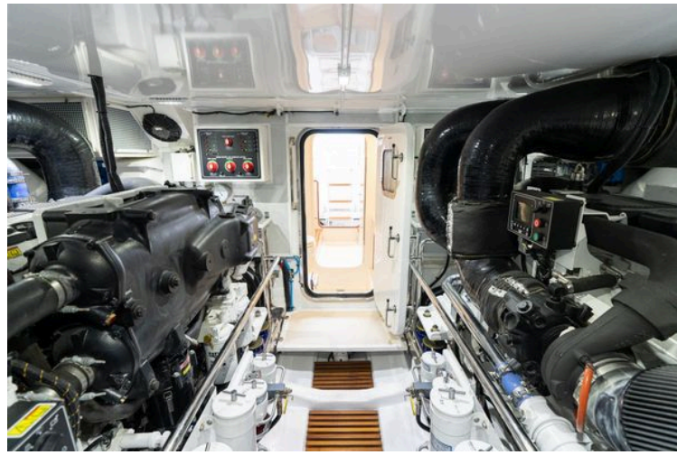
Engine Room Facing Aft
