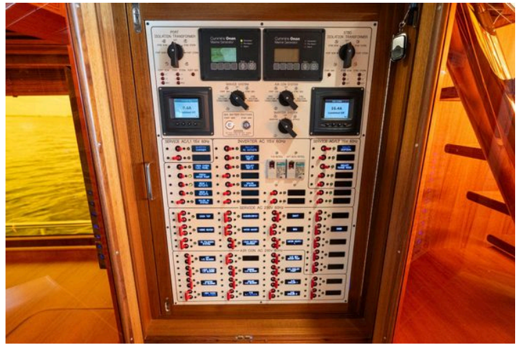
Central Breaker Panel
