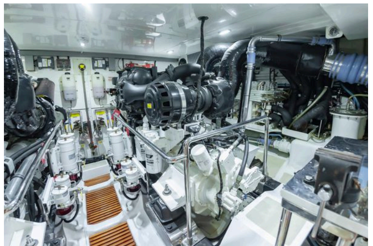
Engine Room Facing Starboard
