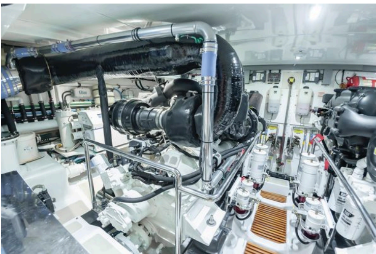
Engine Room Facing Portside
