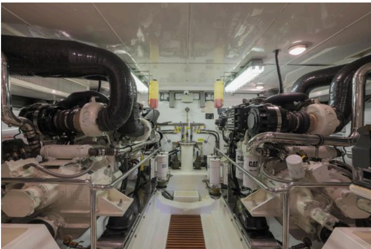
Engine Room Facing Fwd
