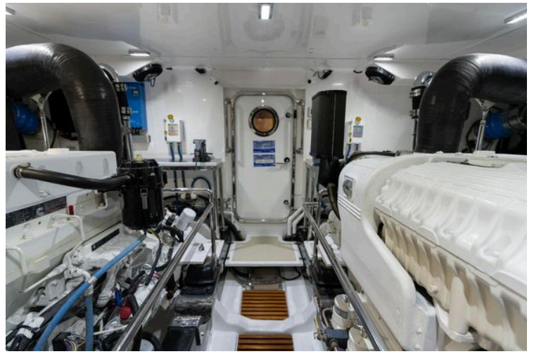
Engine Room Aft
