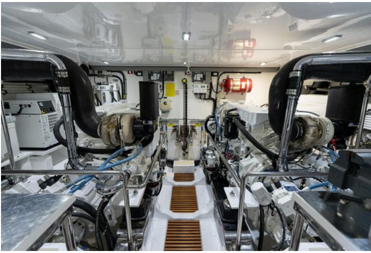
Engine Room Forward
