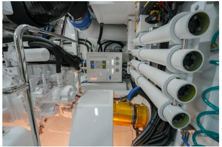
Engine Room Facing Starboard
