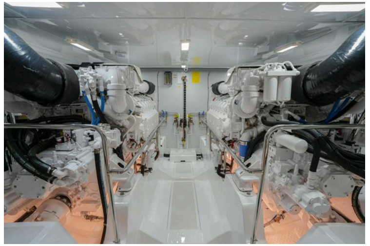
Engine Room Facing Forward
