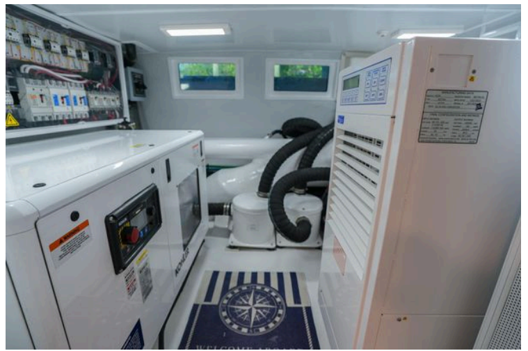
Generator Room Facing Port
