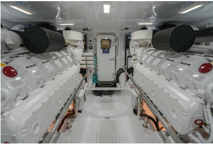
Engine Room Facing Aft
