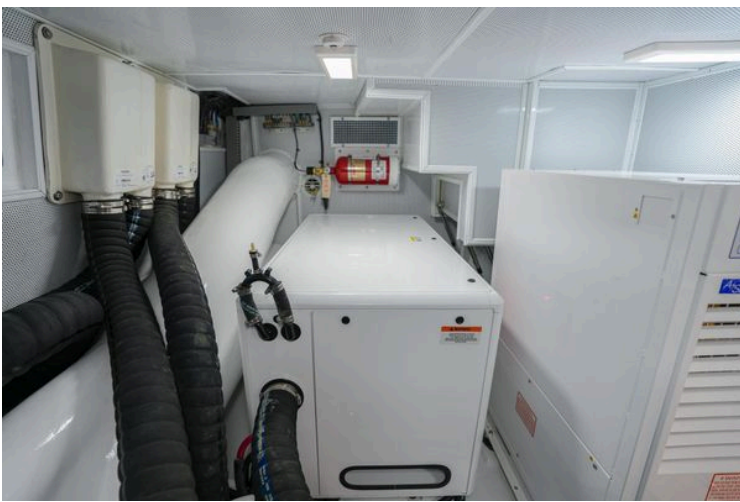
Generator Room Facing Forward
