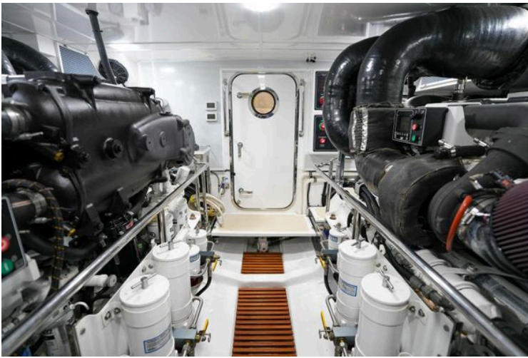
Engine Room Facing Aft
