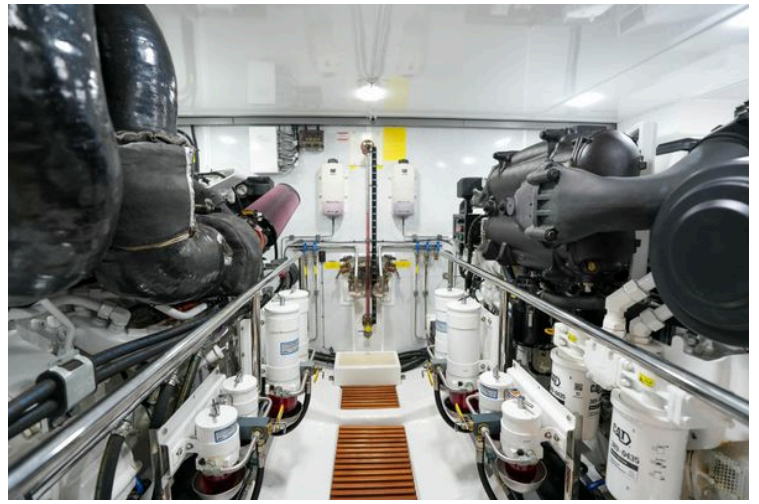
Engine Room Facing Forward
