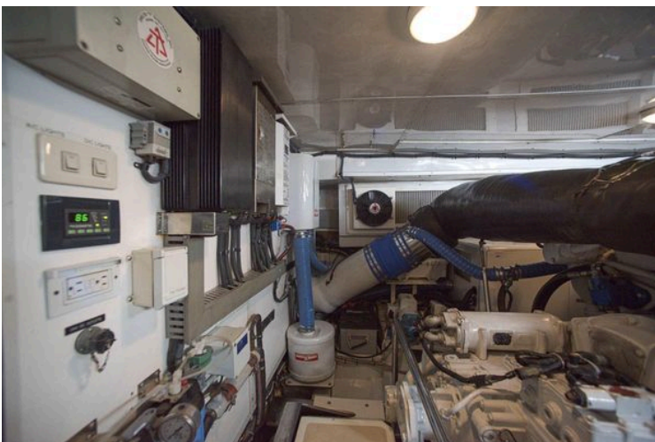
Engine room of 2009 Marlow 78E yacht with control panels and ventilation system.
