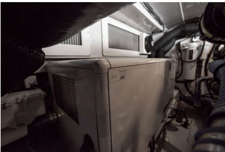
Engine room of 2009 Marlow 78E yacht with visible machinery and ventilation.
