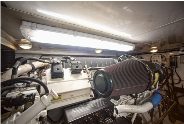
Engine room of 2009 Marlow 78E yacht, featuring mechanical components and lighting.
