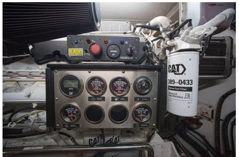
Engine control panel of 2009 Marlow 78E yacht with gauges and CAT marine fuel filter.
