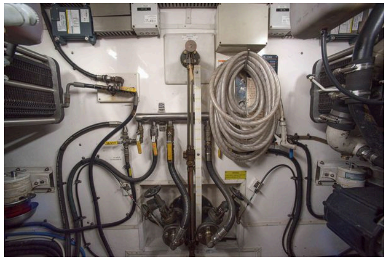
Engine room of 2009 Marlow 78E yacht with hoses and mechanical components.
