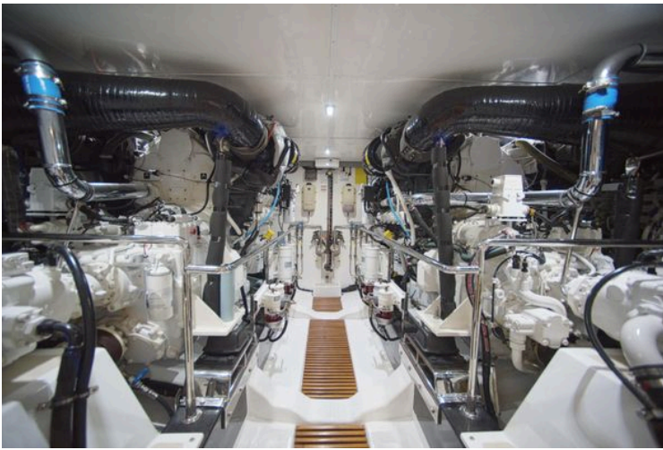
Engine Room Looking Forward
