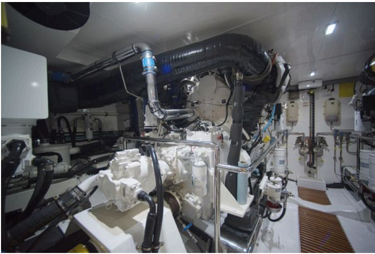
Engine room of 2018 Marlow 75E-CB yacht, showcasing complex machinery and piping.
