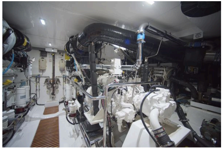
Engine room of 2018 Marlow 75E-CB yacht, showcasing complex machinery and piping systems.
