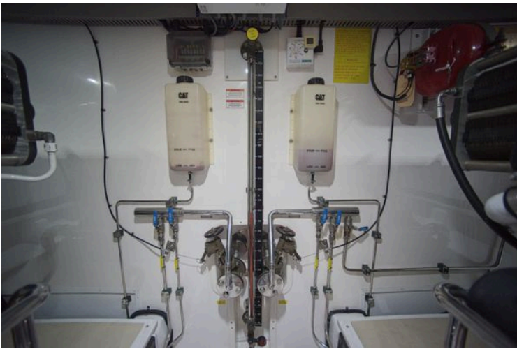
Forward Engine Room Wall, Fuel Manifold
