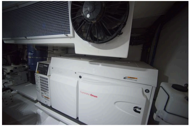
Engine room of 2018 Marlow 75E-CB with Cummins Onan generator.
