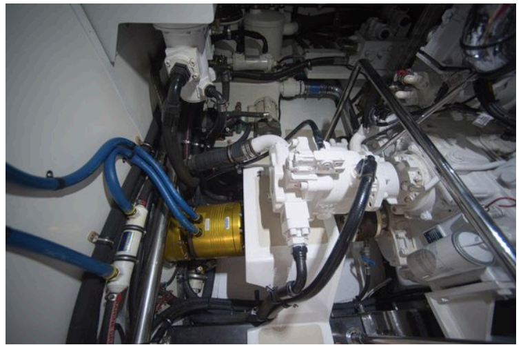
Port Engine Shaft System
