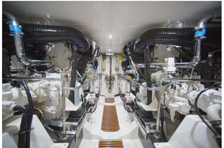
Engine Room Looking Forward
