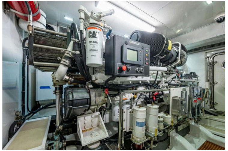
Engine room of a 2013 Marlow Explorer Enclosed Bridge (CB) yacht.
