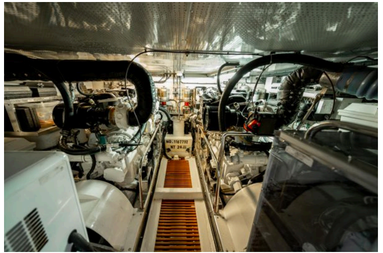
Engine Room Fwd
