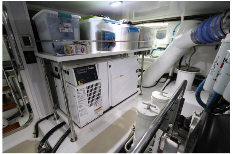
Engine room of 2017 Marlow Explorer 49E with Cummins Onan generator and storage containers.
