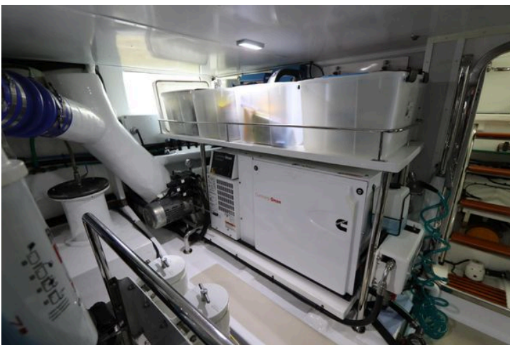
Engine room of 2017 Marlow Explorer 49E yacht with Cummins Onan generator.
