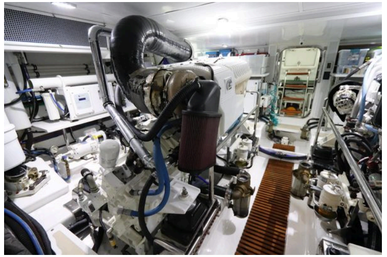
Engine room of 2017 Marlow Explorer 49E yacht, showcasing advanced machinery and equipment.
