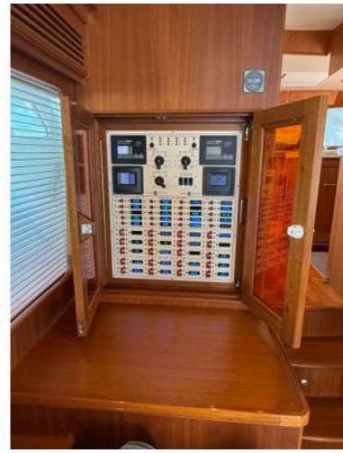
Electrical panel inside 2017 Marlow Explorer 49E yacht, featuring control switches and displays.
