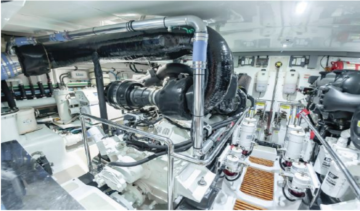
Engine Room facing Portside
