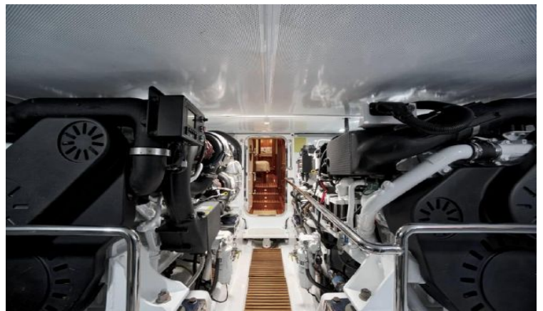
Engine Room Looking Aft
