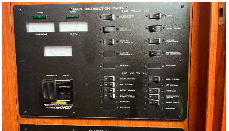
AC power distribution panel
