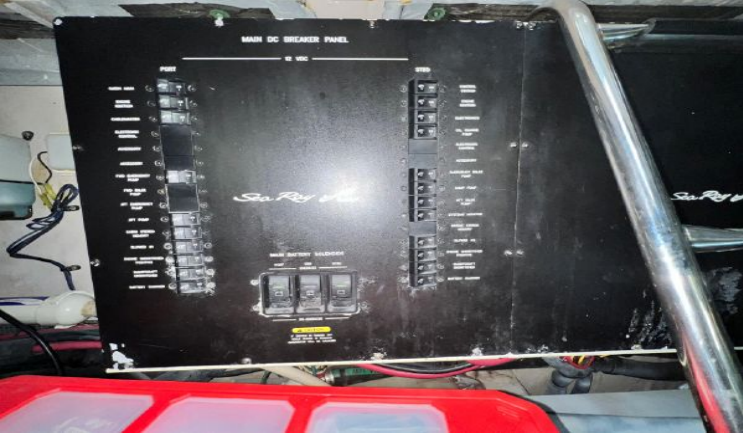
Main DC breaker panel
