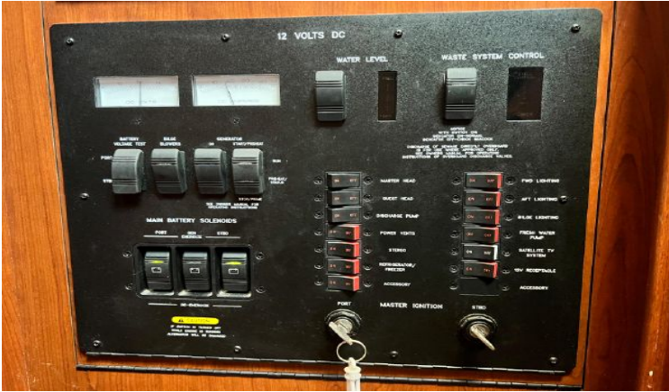
DC power panel
