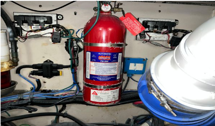
Fire suppressant system
